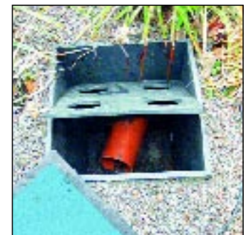
APP eco-inspection boxes controlled drainage in the planting area
